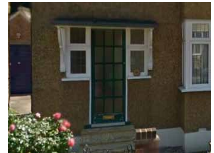
Flat or pitched canopies (on brackets). The example is a flat canopy over a door with side lights
