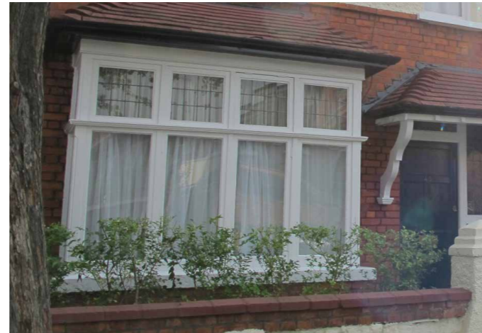
Edwardian projecting square timber bay windows with casement opening and leaded transom lights
