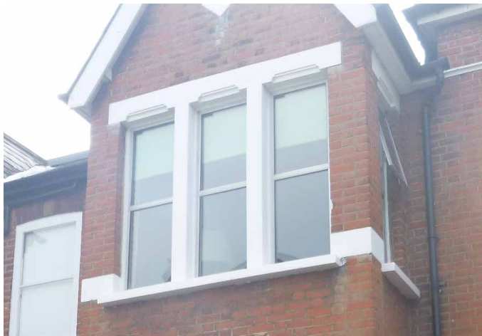
Replacement narrow bar uPVC windows filling three long openings in a late-Victorian bay
